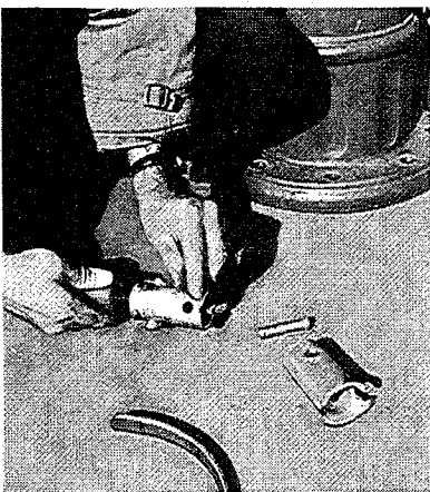
7. SAFETY STEM COUPLING SHOULD BE INSTALLED WITH NOTCHES TOWARDS THE LOWER STEM. WORDS "THIS END UP" TOWARDS THE UPPER STEM.
