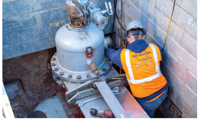
FIGURE 1 - CONTRACTOR, TAP MASTER INC., INSTALLING THE PERMASEAL INSERTION VALVE FOR THE CITY OF PHOENIX WATER SERVICE DEPARTMENT BY UTILIZING MUELLER CL-12 AND C1-36 DRILLING MACHINES FOR CUTTING AND VALVE INSERTION OPERATIONS.
